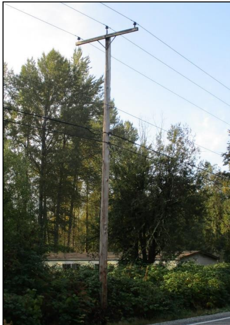
12kV Distribution Line
