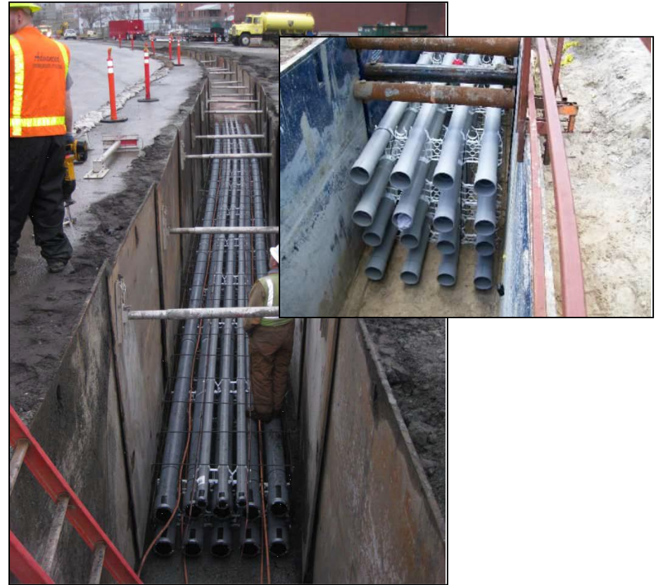
Cable Duct Bank
