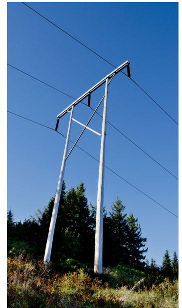
230kV transmission lines
