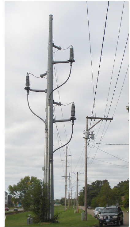
Example of a steel underground termination structure. Photo courtesy of POWER Engineers, Inc.
